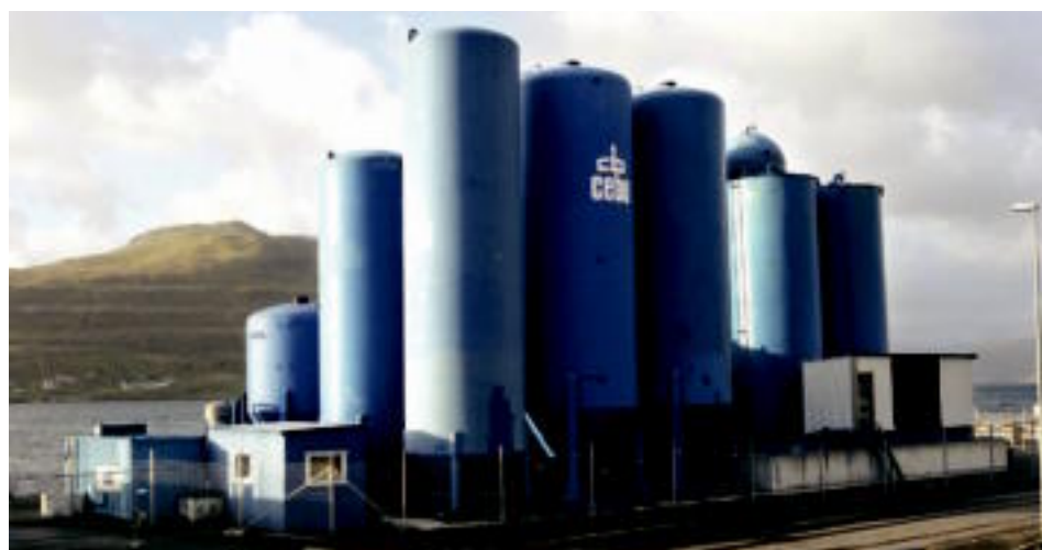
Bulk and Mud Plant
